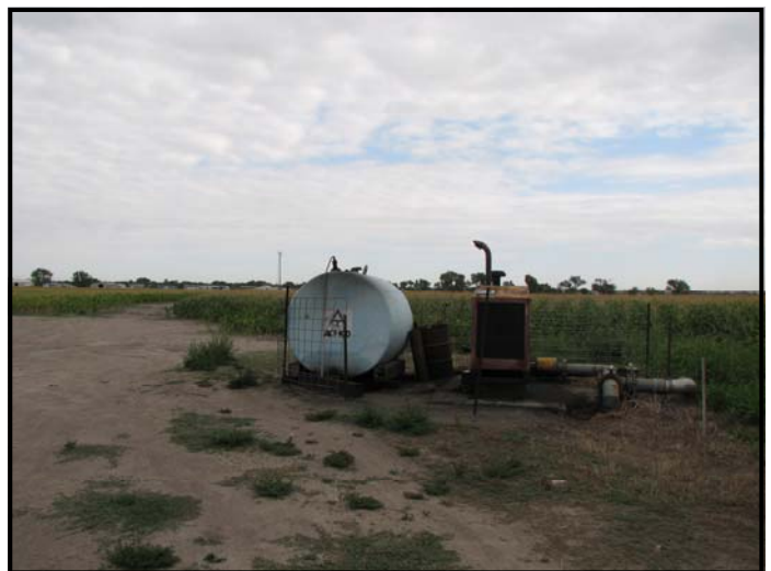
Diesel Power Unit Parcel #2
